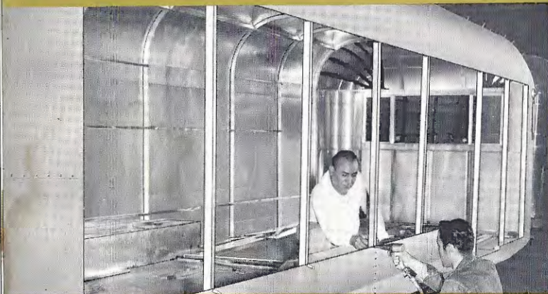
The ribs are placed in position and the sides are being riveted on.
