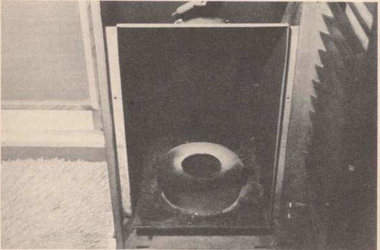
Sooty fire boxes cause oil heater to operate inefficiently. At least once a year, clean out soot, ash, carbon and other residue.
