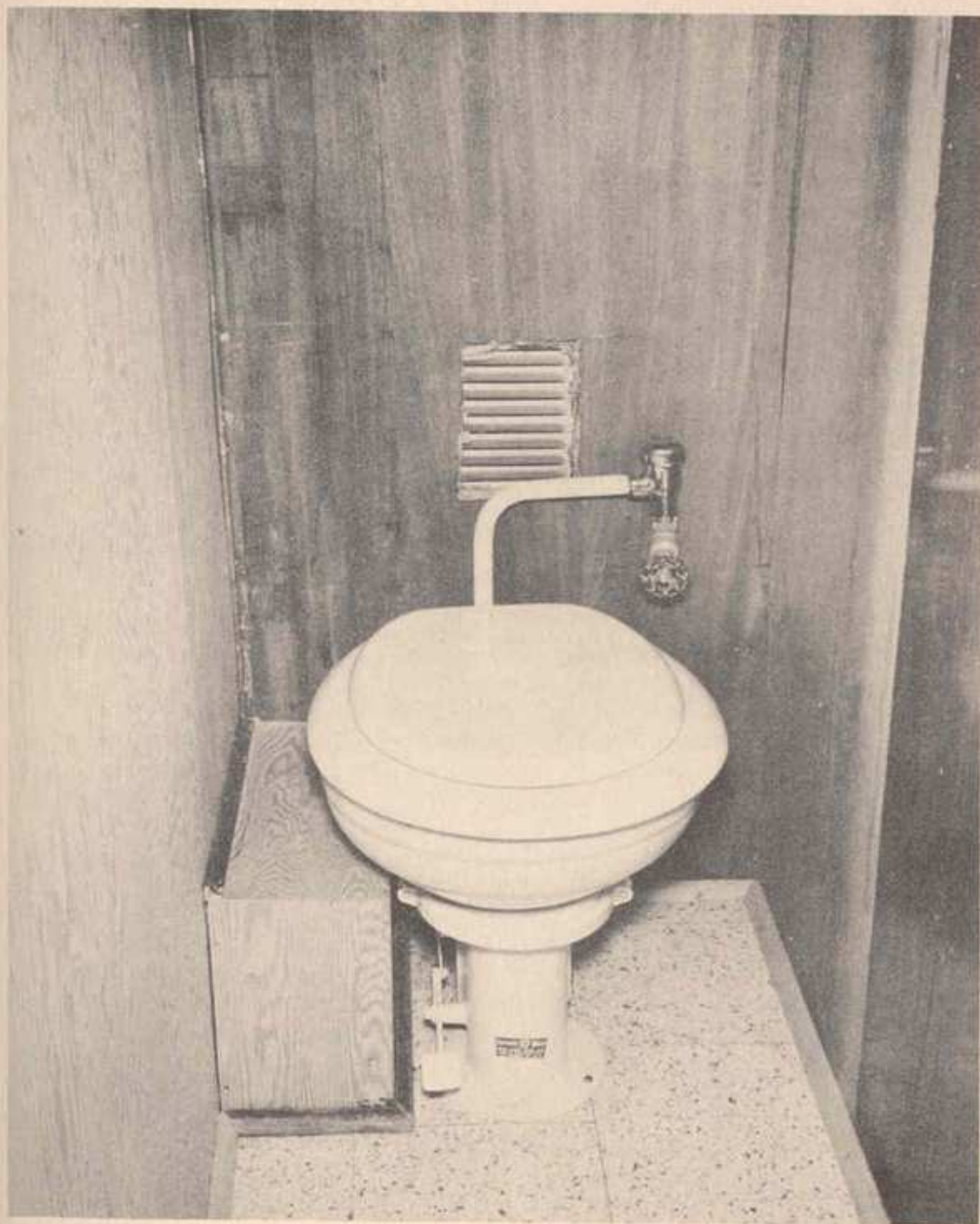
Picture 9. Building in bathroom is under way. Floor plan did not allow for tub or shower. Toilet is in. Wash basin is to be installed.
