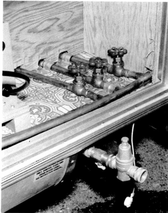
Drain Valves in Converter/Battery Charger Compartment
