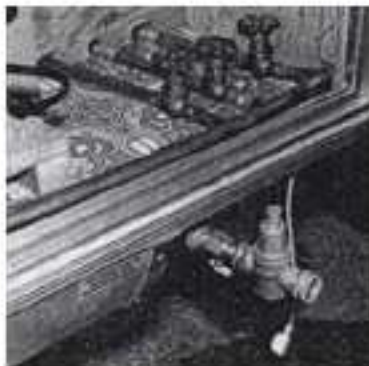
Drain Valves in Converter/Battery Charger Compartment
